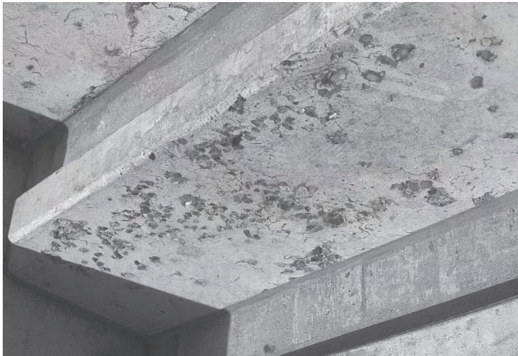
Figure 5.18 Surface pop-outs caused by microporous flint aggregate in the concrete.
