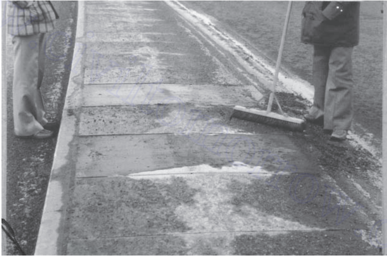
Figure 5.19 Scaling of a concrete surface owing to freeze–thaw, exacerbated by de-icing salts.
